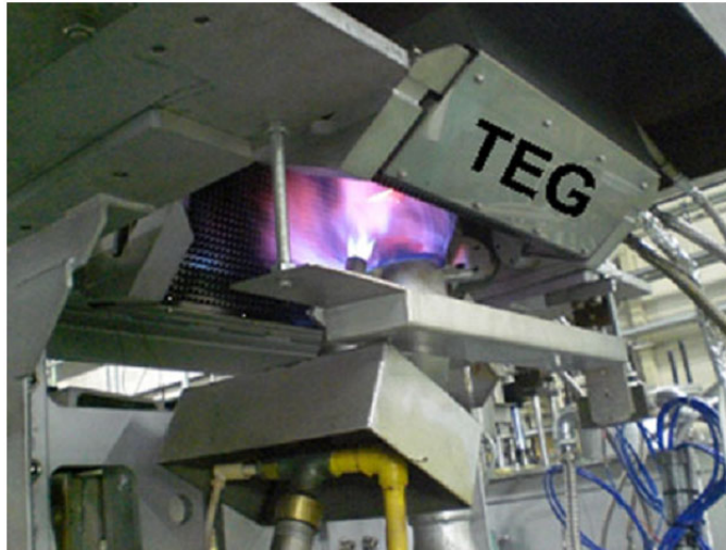
Fig. 4. Installation of thermoelectric generator on cement kiln of the Awazu plant of company Komatsu (Japan) [31].
