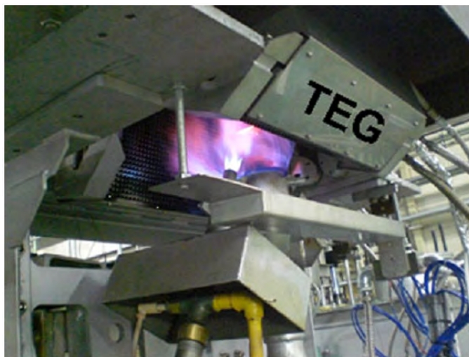
Fig. 4. Installation of thermoelectric generator on cement kiln of the Awazu plant of company Komatsu (Japan) [31].
